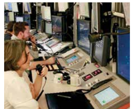
Strasbourg: IFR approach room and FIS position in the new tower.
