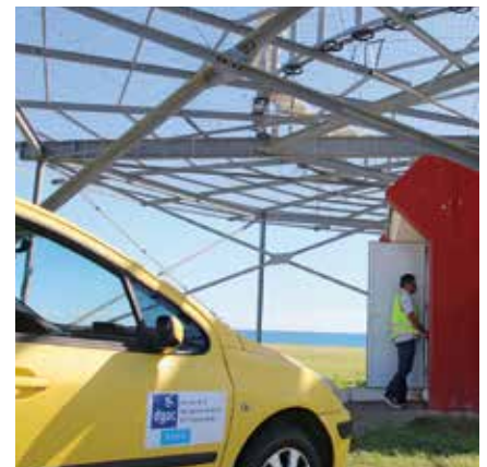
VOR maintenance visit at the Saint-Denis airport in La Reunion.
